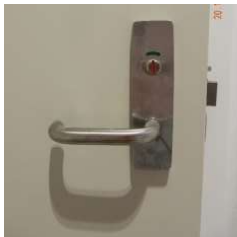
The above image indicates a privacy latch set provided to accessible WC facilities as viewed from the outside
